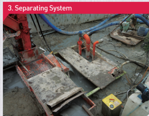
1st cleaning by desander with rock fragments and soil materials on the surface
