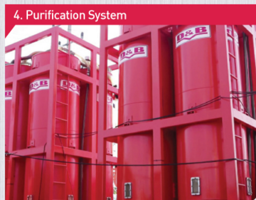
2nd cleaning by purification system for suspended solid and fine particles
